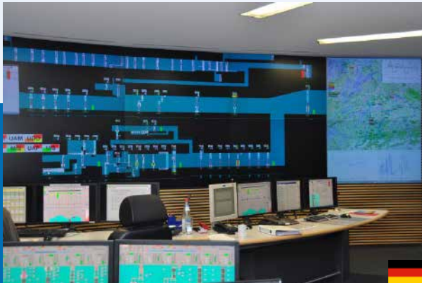
E.ON dispatch center Landshut
